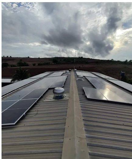
ROOF • SOLAR AT DUSK
